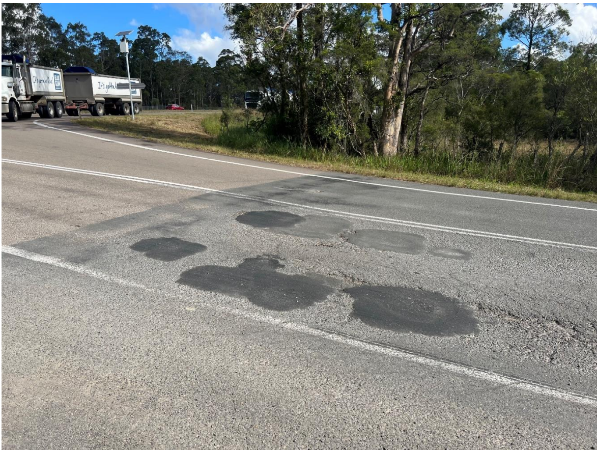
Figure 3.2 Road surface defects on Italia Road near the intersection, looking south
